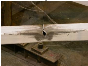
c) Fracture of brace
