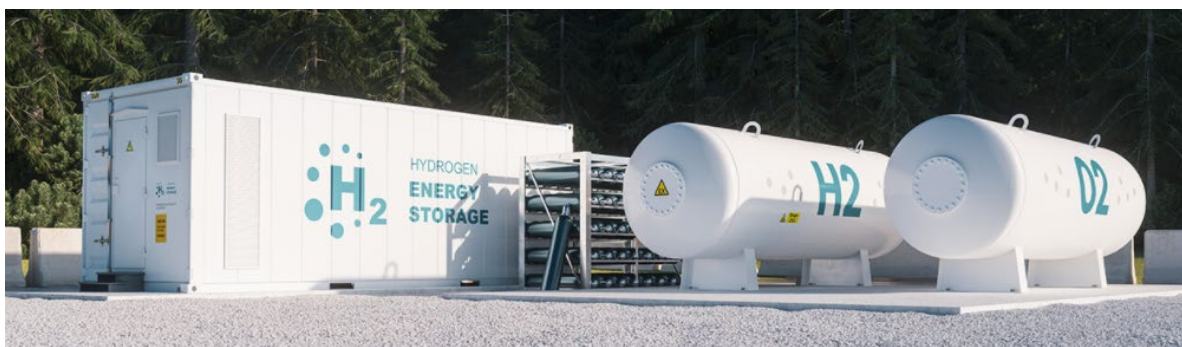
Fig.1: Example of a high-pressure storage tanks – bullets (left) and bottles (right).
